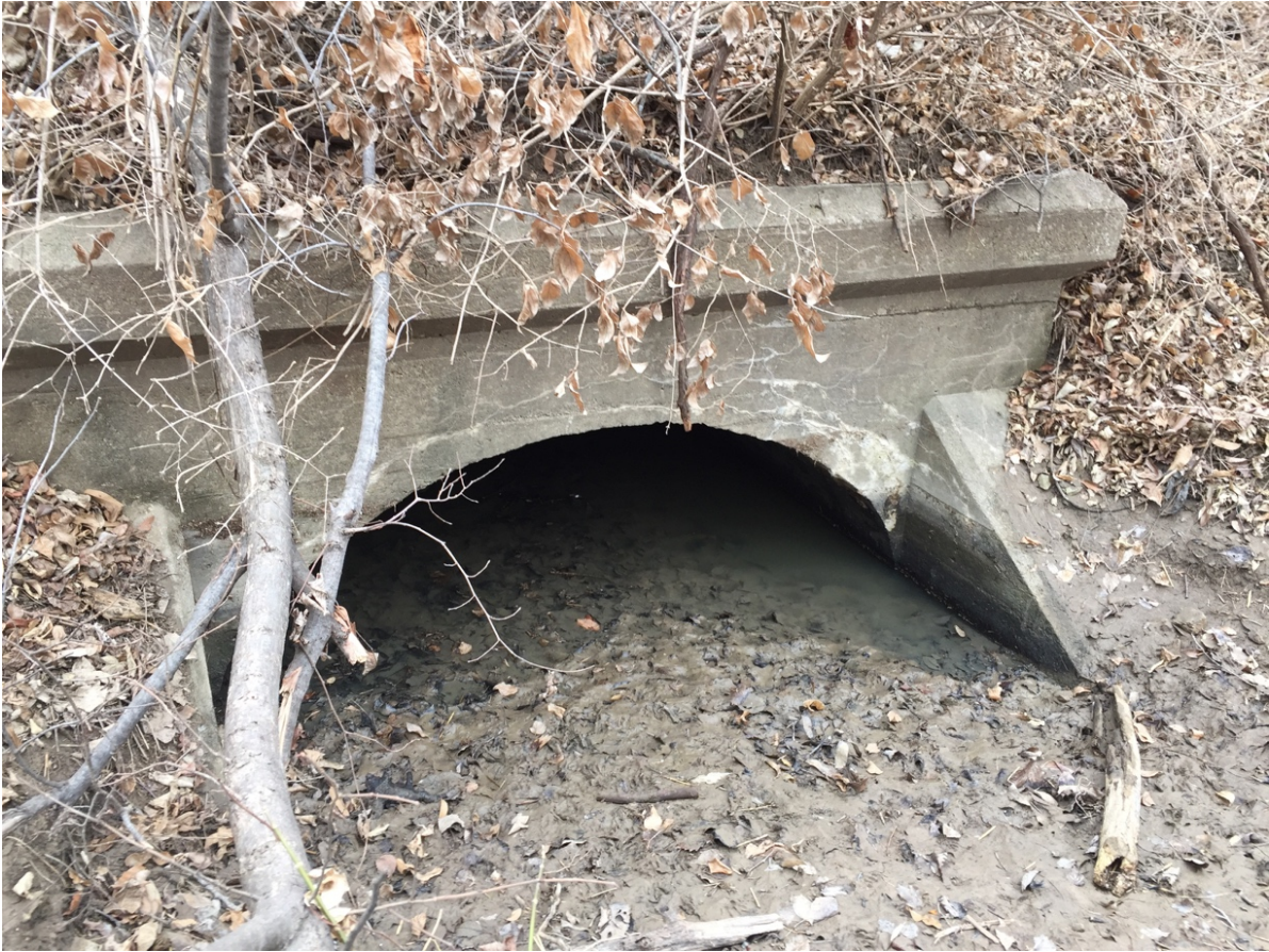
Culvert at MP 286.5, Kansas City. General view of west façade looking southeast. Date: February 7, 2017
