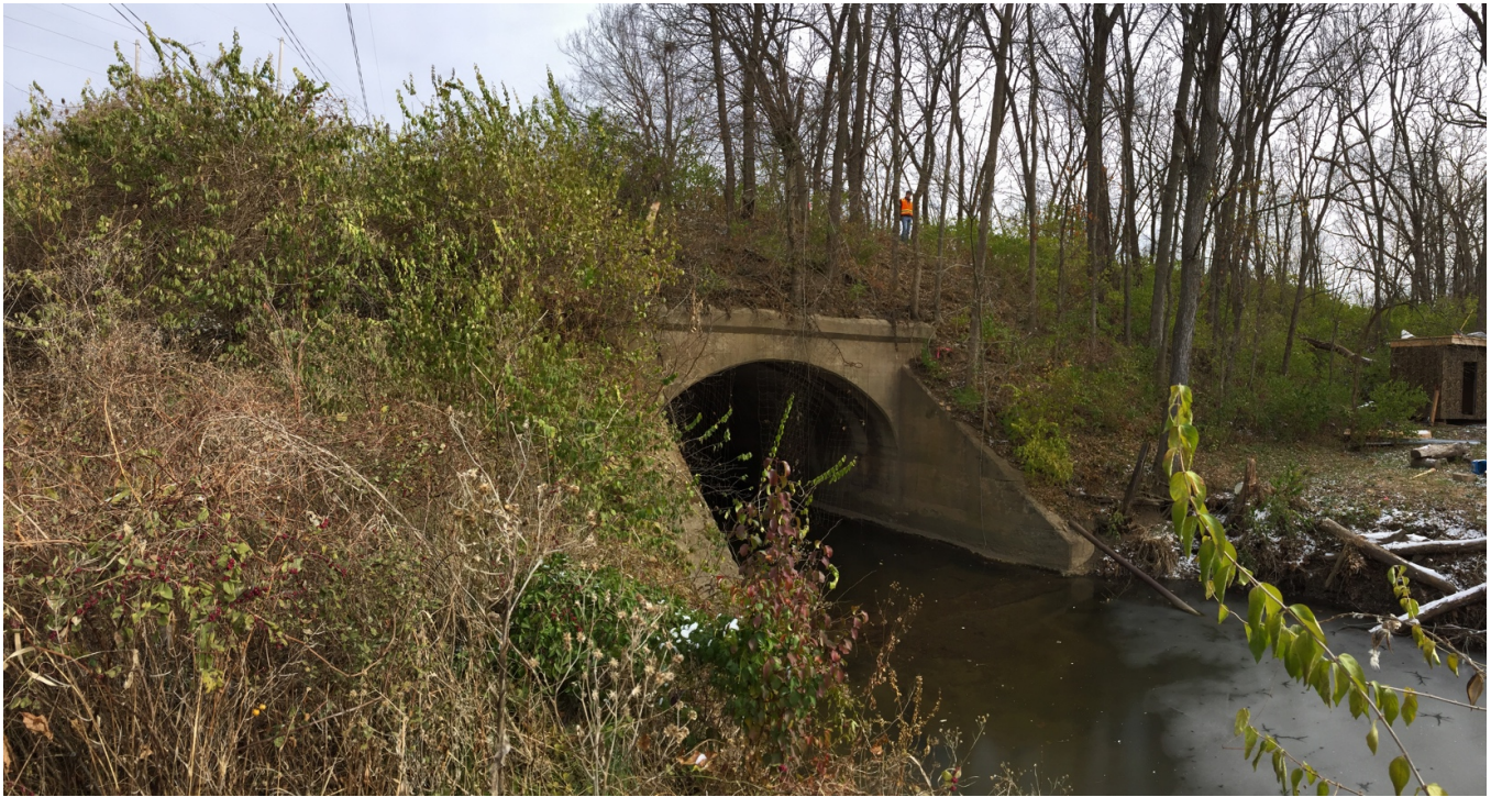
Culvert at MP 273.5, Lee's Summit. General view of the west façade, looking southeast (above); General view of the west façade, looking east (below). Date: December 9, 2016
