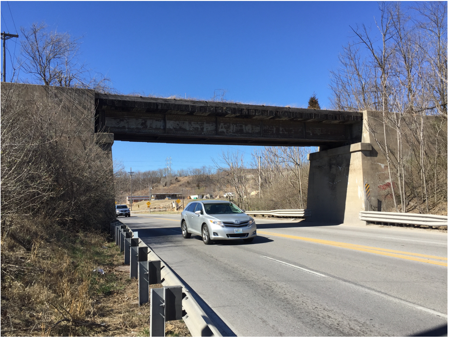
Bridge at MP 279.0 at MO Highway 350. View of the south façade, facing northeast. Date: March 7, 2017.
