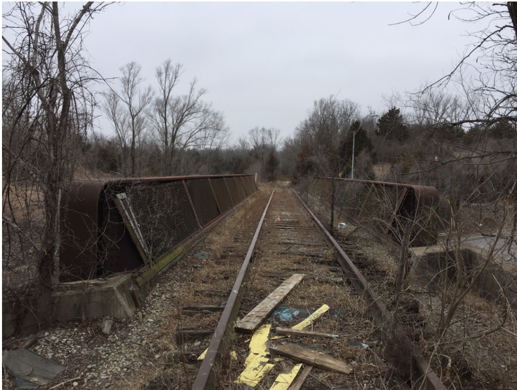
Bridge at MP 285.2, Raytown, MO. General view of the deck; view facing west (above); general view of the tracks and deck; view facing east (below). Date: February 7, 2017.
