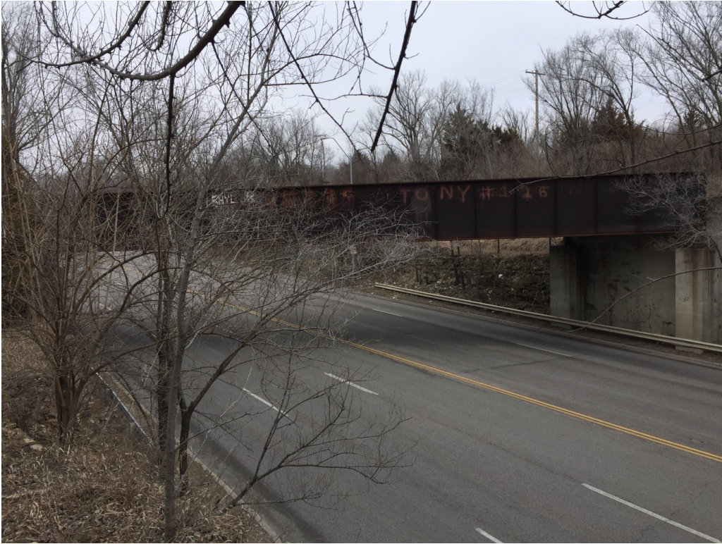
Bridge at MP 285.2, Raytown, MO. General view of the south façade; view facing north (above); general view of the south façade; view facing northeast (below). Date: February 7, 2017
