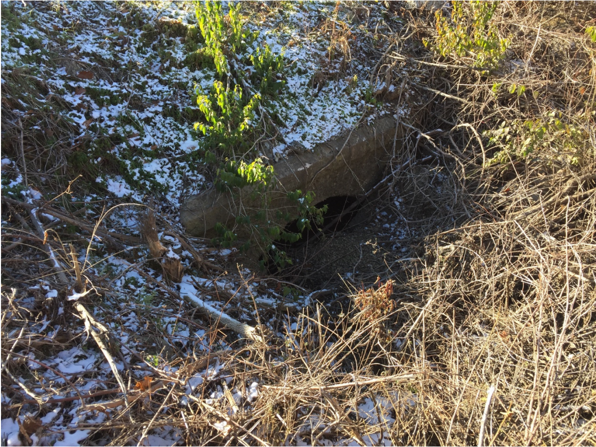
Culvert at MP 272.2, Lee's Summit. General view of the east façade looking northwest. Date: December 9, 2016.
