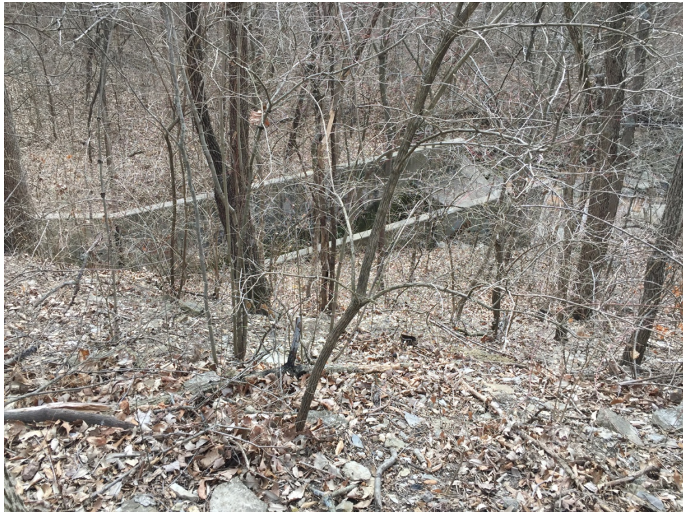
Culvert and Flume at MP 286.2, Kansas City. General view facing east, southeast (above); view from rail corridor facing southwest (below). Date: February 7, 2017
