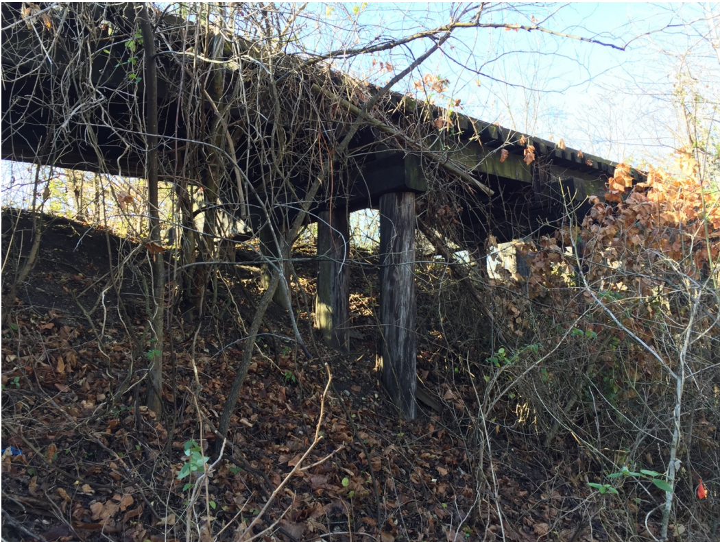
Bridge at MP 281.5. General view of the east façade, looking northwest (above) and a detail of the substructure, looking northwest (below). Date: December 5, 2016
