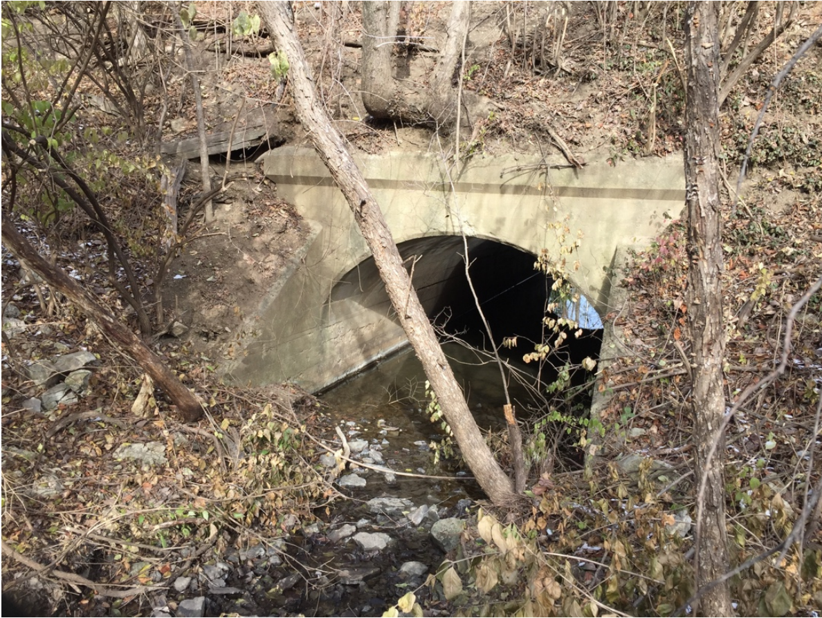
Culvert at MP 273.1, Lee's Summit. General view of the west façade looking northeast. Date: December 9, 2016
