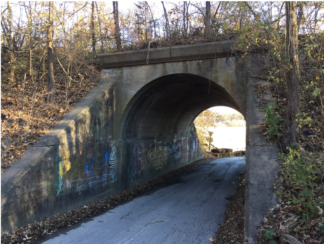
Bridge at MP 280.00 over Frost Road, Raytown, MO. General view of the west façade (above) and east façade (below). Date: December 6, 2016
