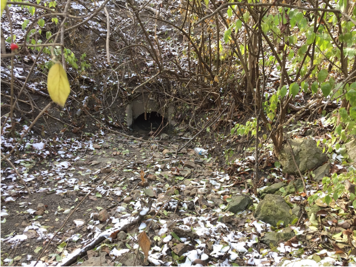
Culvert at MP 273.5, Lee's Summit. View of the west façade looking northeast. Date: December 9, 2016
