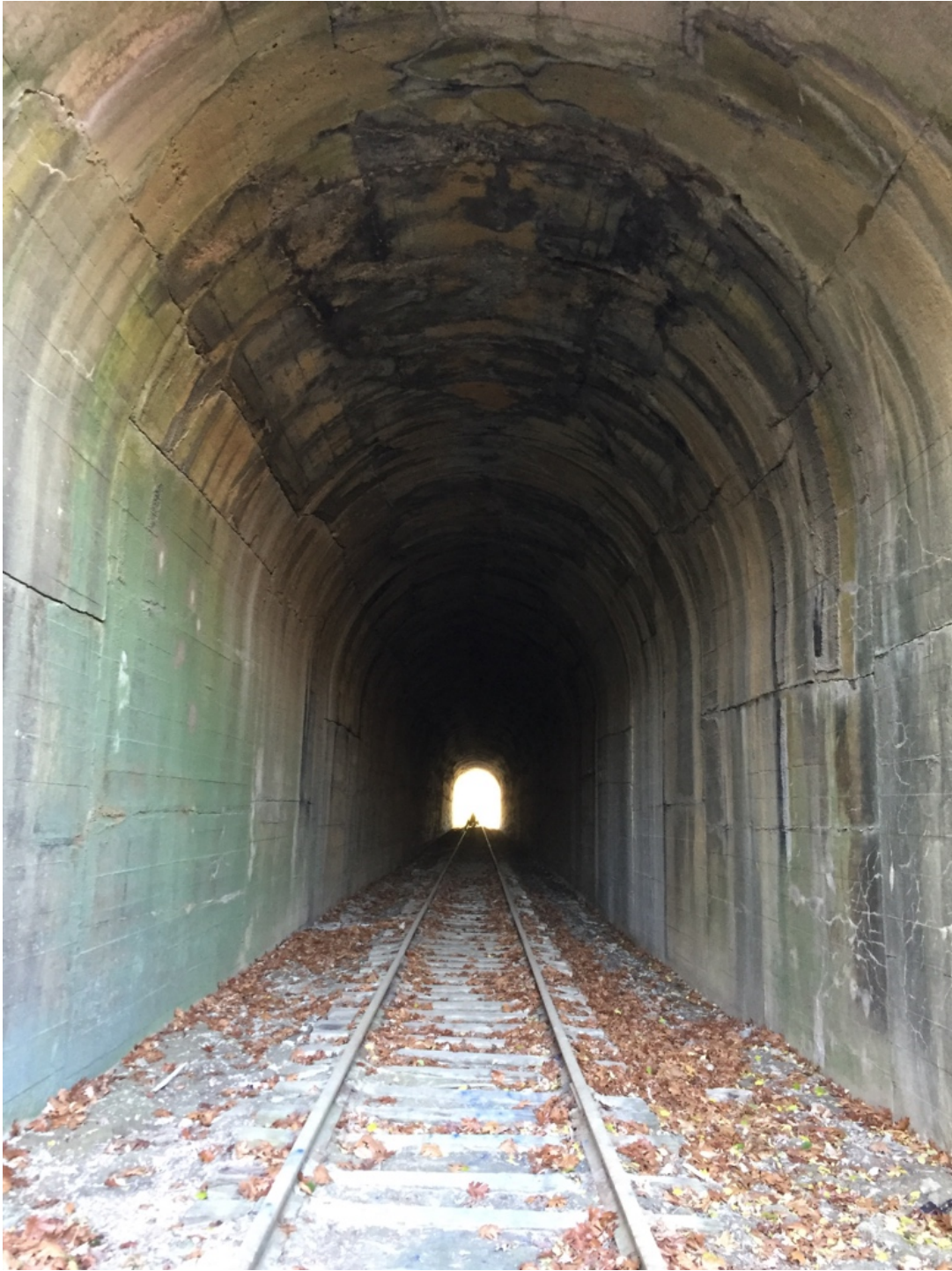
Vale Tunnel at MP No. 277.7. View of the interior, facing south. Date: December 6, 2016
