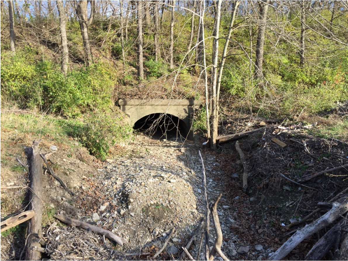
Culvert at MP 276.7, Lee's Summit. General view of the west façade, looking east. Date: December 6, 2017
