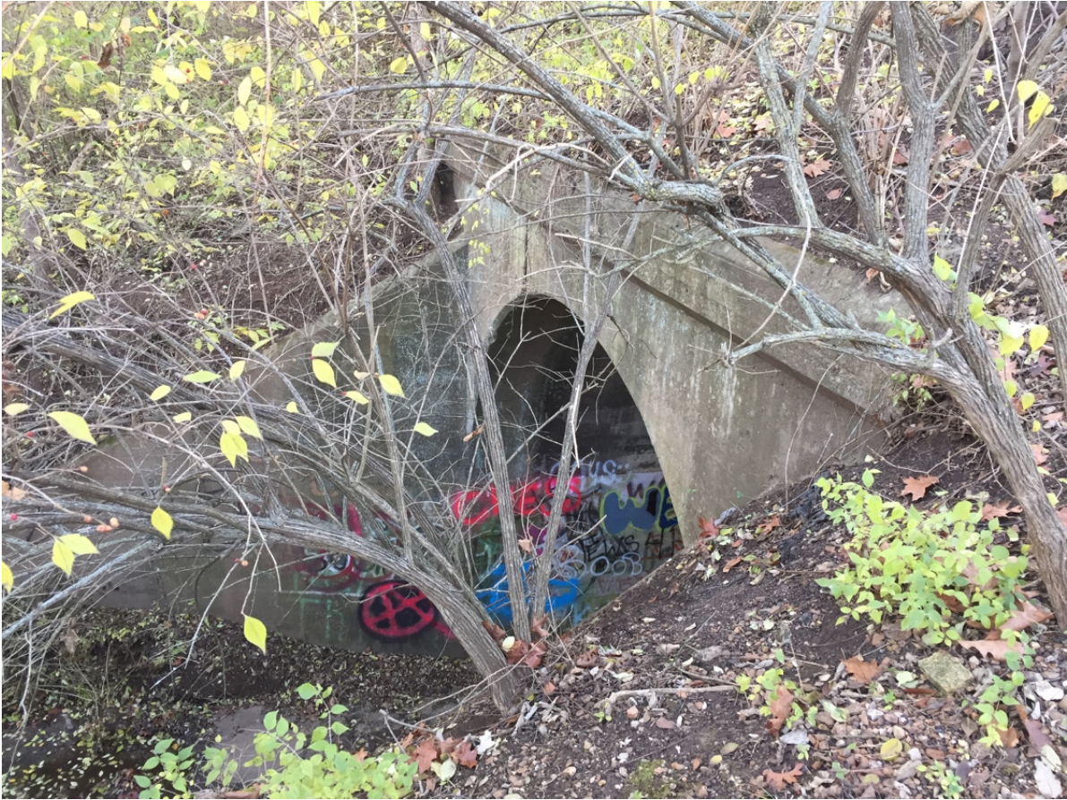
Culvert at MP 274.5, Lee's Summit. General view of the west façade, looking northeast. Date: December 6, 2016
