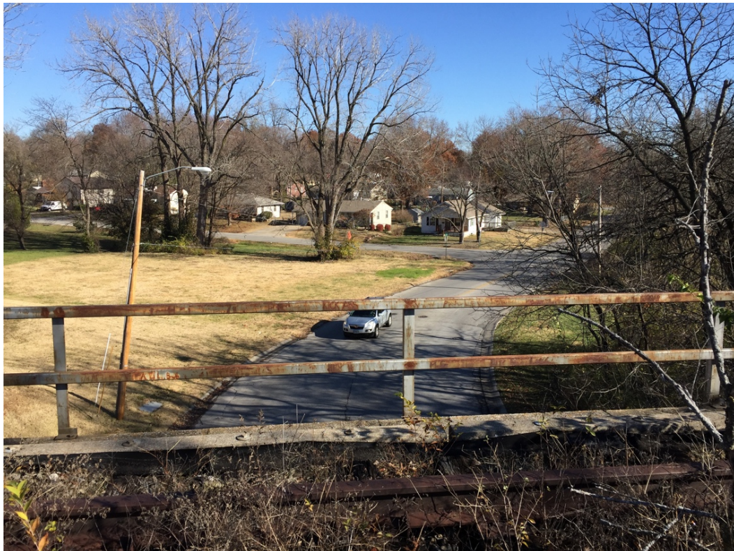
Bridge at MP 282.5. General view of the west façade (above) and a detail of the deck and rail (below). Dates: March 6, 2017 and December 5, 2016.
