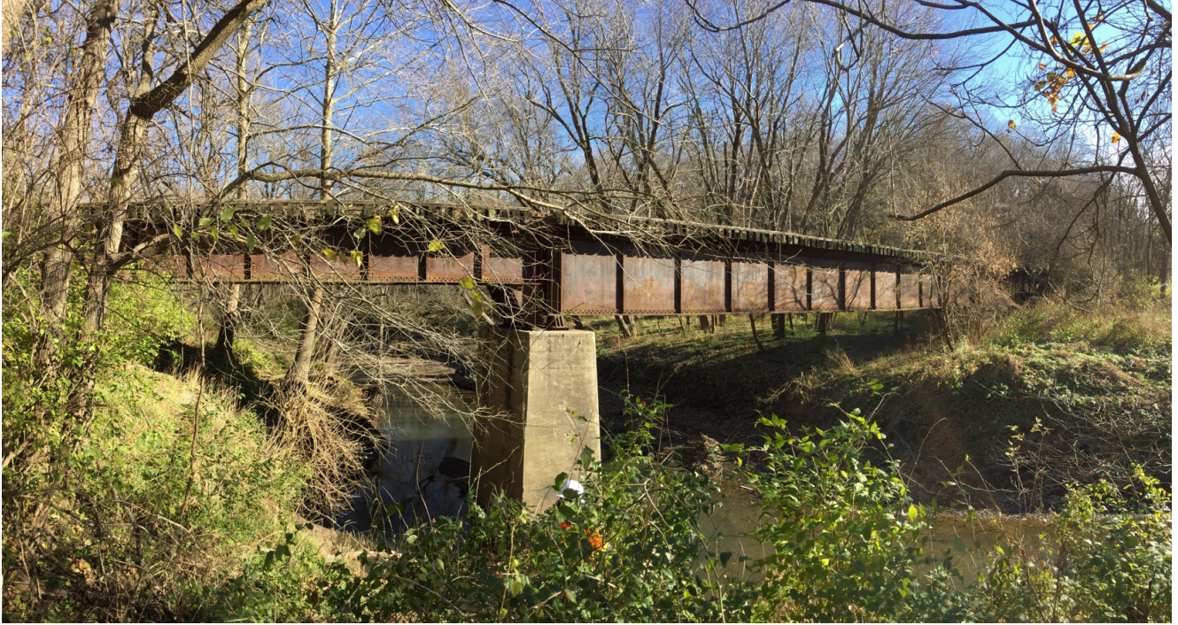
Bridge at MP 277.0 over the Little Blue River. Panorama of the west facade facing southeast (above); Detail of the west façade, looking east (below). Date: December 6, 2016.
