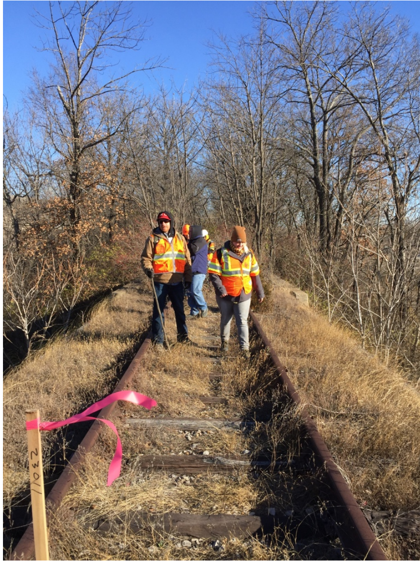
Bridge at MP 279.0 at MO Highway 350. View of the tracks on the deck of the bridge, facing east. Date: December 6, 2016.
