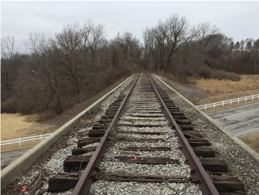
Bridge No. 285.5, Kansas City, MO. General view of the east façade, facing northwest (above); View of the deck facing north (below). Date: February 7, 2017
