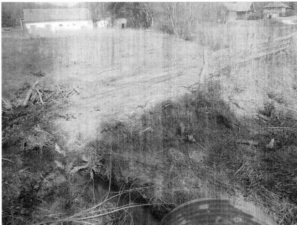
Photo 2. NRPW 2 at Lee's Summit Road Crossing
