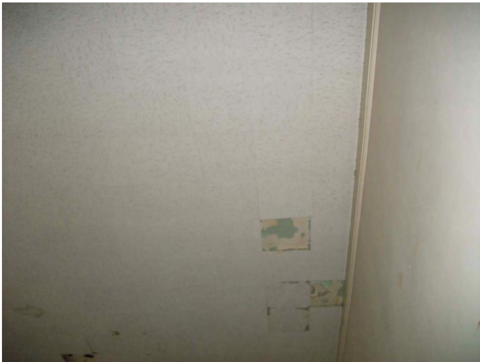
Homogenous Area V – 1x1 Ceiling Tile
