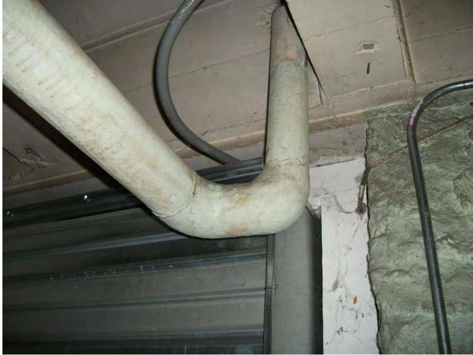
Homogenous Area I – Muddied Joint Packing on Air Cell Pipe Cover
