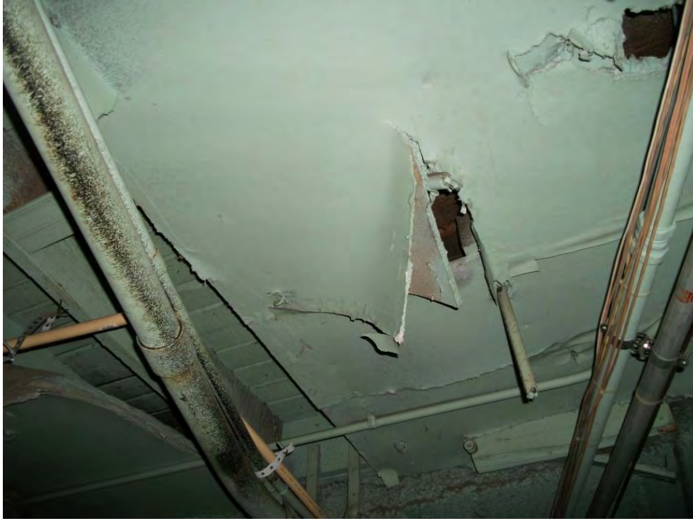
Homogenous Area G – Asbestos Board
