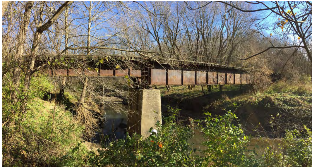
Panoramic view of a deck plate girder bridge over the Little Blue River, north of I-470; looking east.
