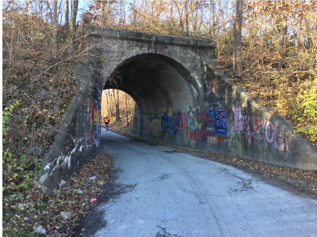
Skewed concrete arch bridge at Frost Rd. and east 79 th St.; view looking northeast.
