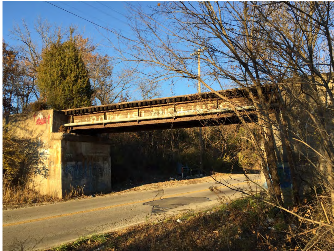
Deck plate girder bridge at 47 th St. and Raytown Rd.; view looking east northeast.
