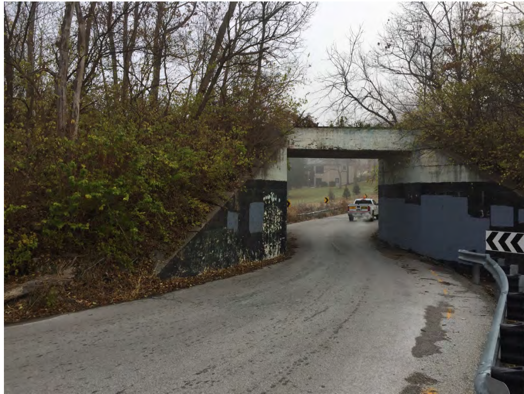
Concrete skewed bridge at 75 th St. between Westridge Rd. and Larson Ave.; view looking northwest.
