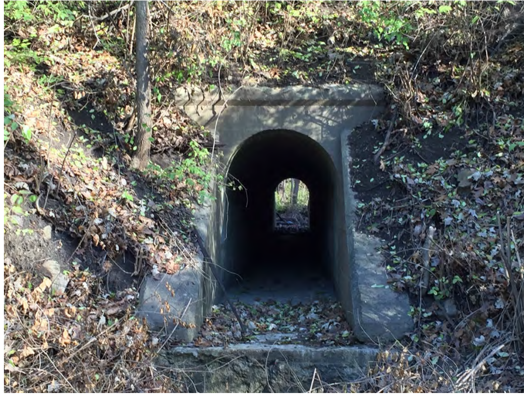
Concrete arch culvert north of NW Chipman Rd.; view looking east from the right-of-way.
