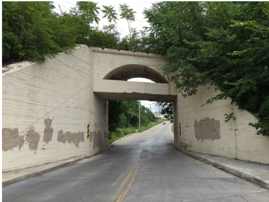
Skewed concrete arch bridge at Raytown Rd. and Stadium Dr.; view looking east.
