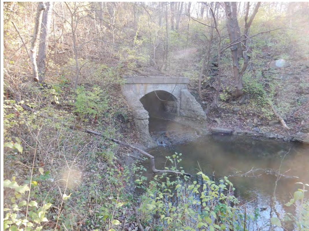
Concrete arch culvert near Blue Ridge Cutoff and East 47 th St. (KML 111)
